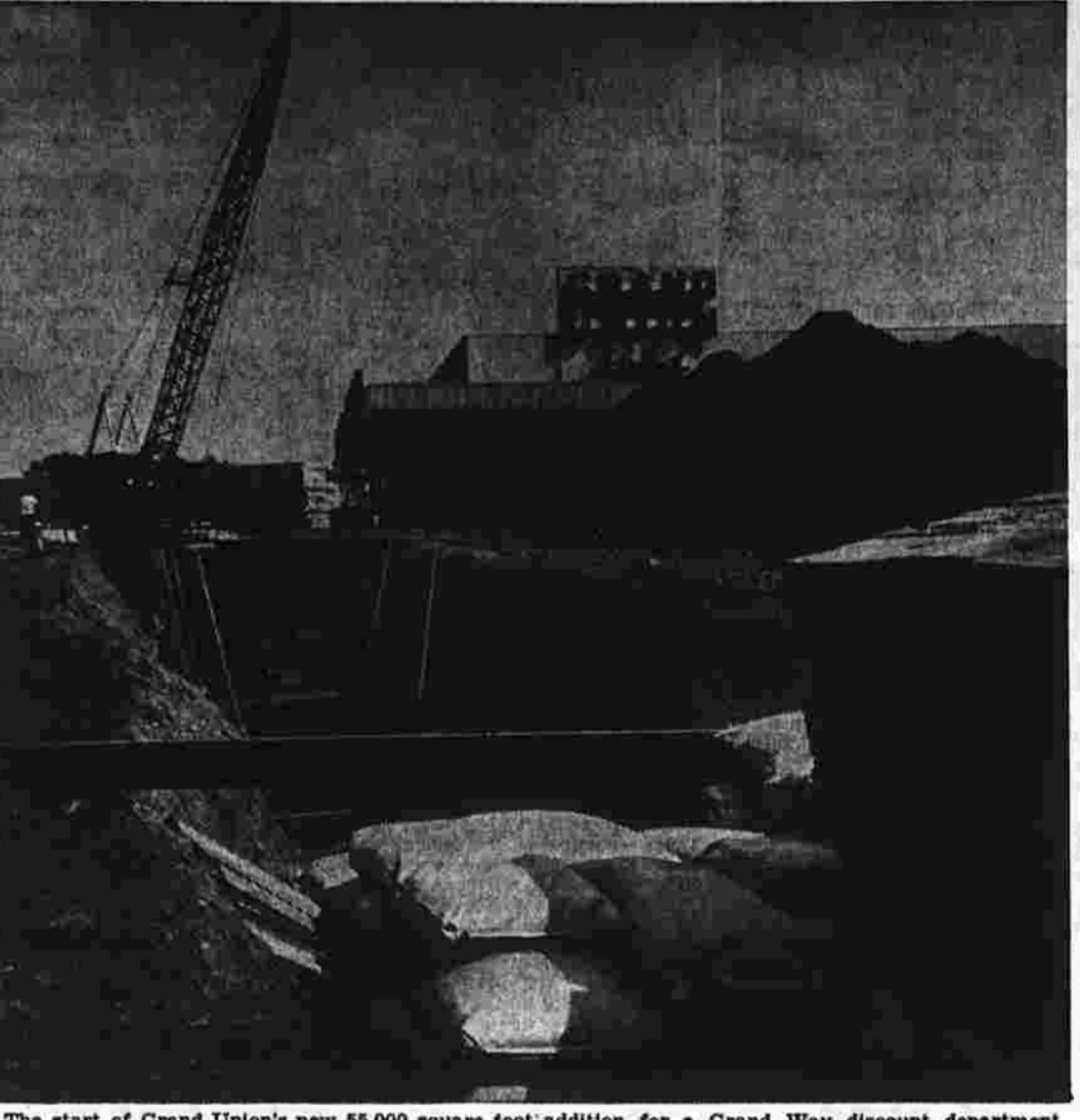
The start of Grand Union's new 55,000 square foot addition for a Grand Way discount department store operation, began this week at the Parkade Shopping Center. Green Manor Const. Co., building the addition here, is laying sanitary sewer lines in the first phase of construction. The newest addition to the Parkade Shopping Center is expected to be completed by Oct. 15. Neil H. Ellis, president of Green Manor Const. Co., said yesterday. (Herald photo by Pinto)
